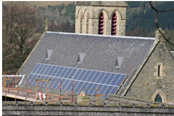
A solar pv system on Selkirk Parish Church. 323
